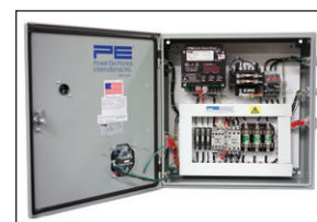
Panel de control
